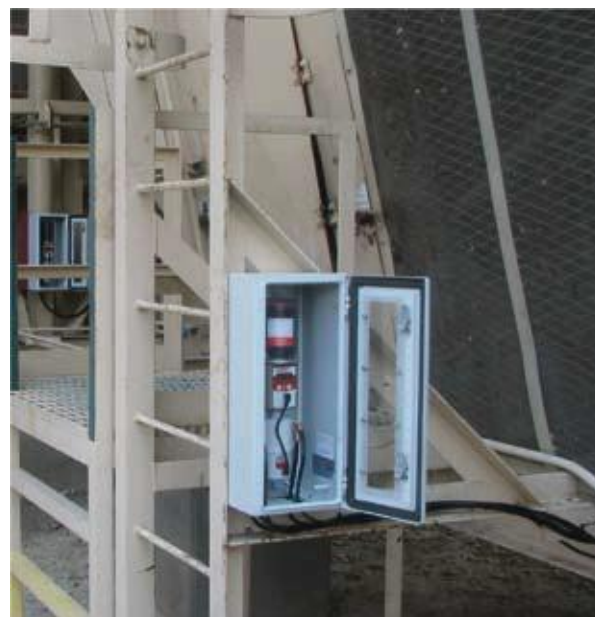
perma PRO MP-6 mounted in enclosure box on gas compression engine cooling fan.
