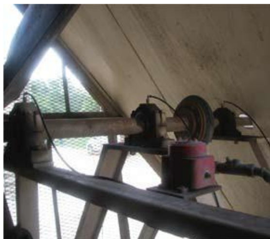
Gas engine compressor fan. Three middle bearings shown with perma 90° tube adapter and 5/16" tubing that is run from externally mounted perma PRO MP-6 automatic lubricators.
