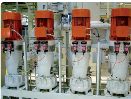
Lubrication system: 2 perma STAR CONTROL 120 cm 3 each
